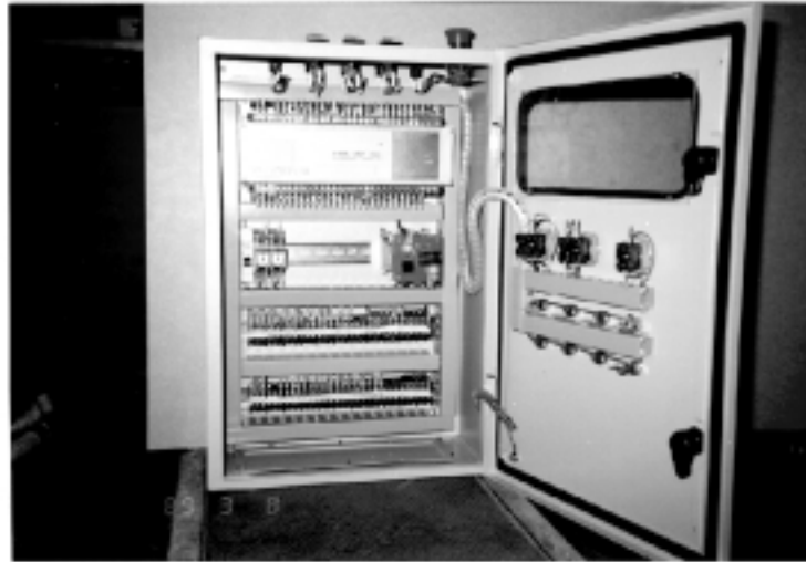
Typical PLC Control Panel
